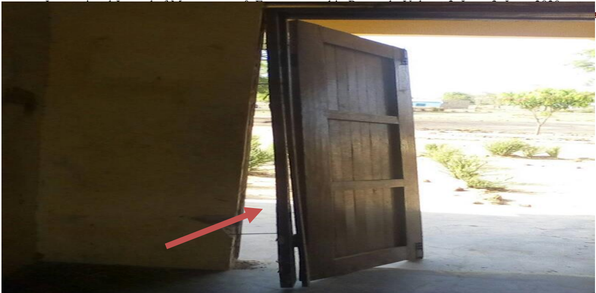
Figure 3e: Plate 5: Damaged Doors of one of the classroom block at Wa Community Development Institute
