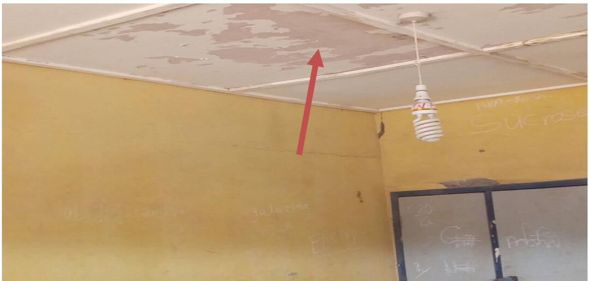
Figure 3d: Plate 4: Discoloring ceiling of one of the offices in the Administration block at Wa Islamic SHS
