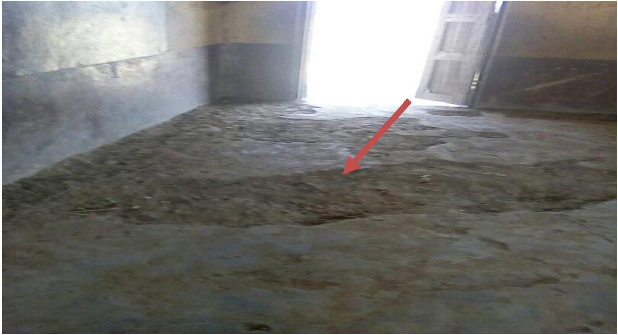
Figure 3g: Plate 7: Cracked on floors and Floor-peeled-off of one of the classroom block at Wa Northern Star Senior High School
