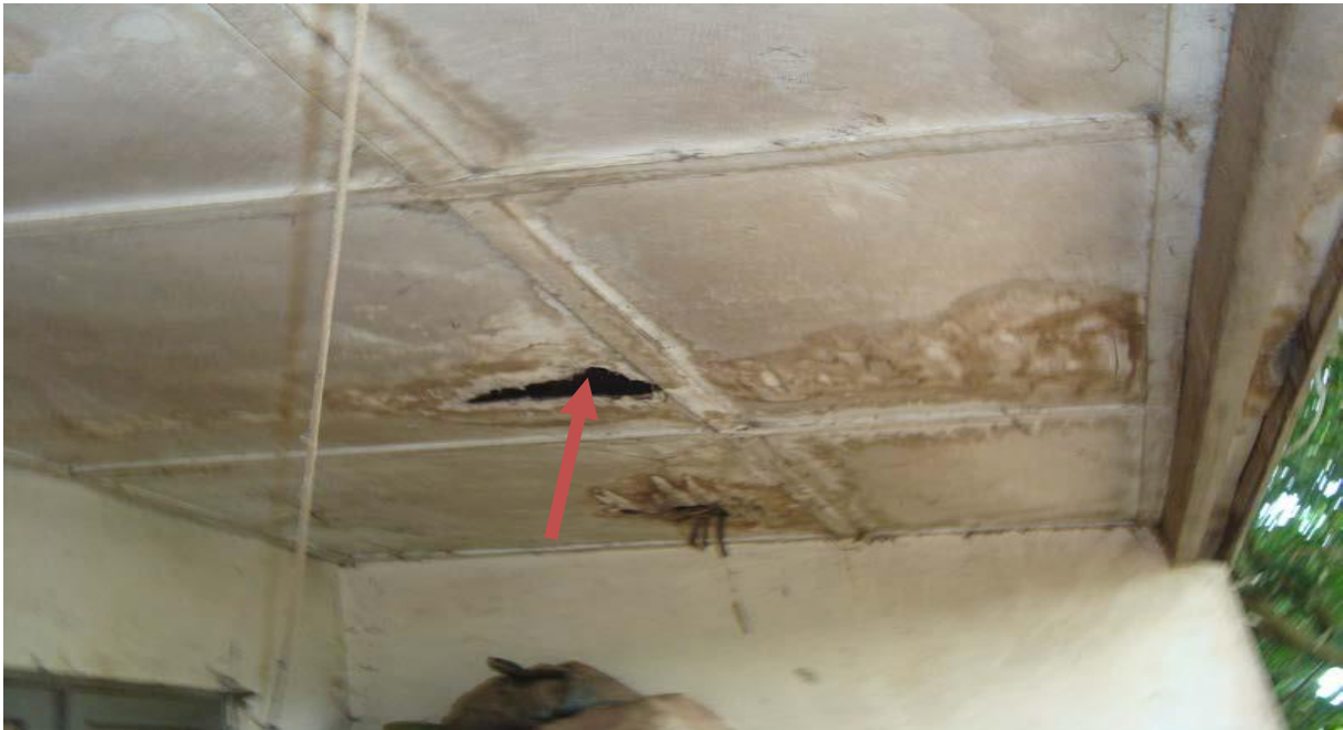
Figure 3f: Plate 6: Damaged Ceiling of one of the classroom blocks at Wa Islamic Girls Senior High School
