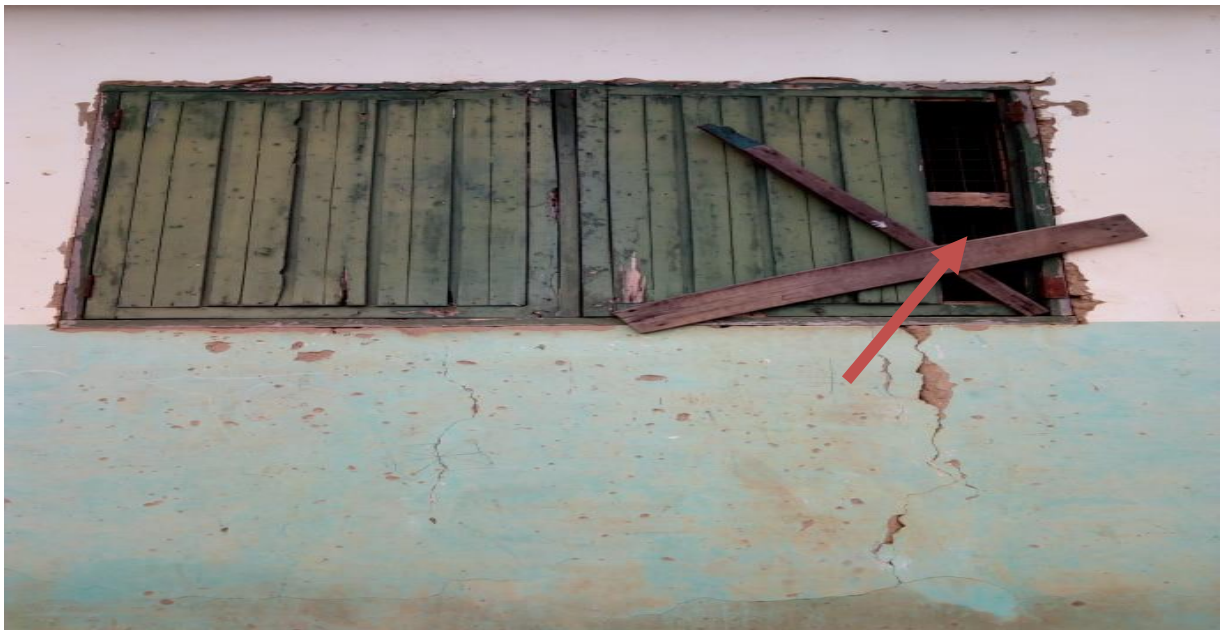
Figure 3b: Damaged classroom windows at Wa Senior High Technical School
