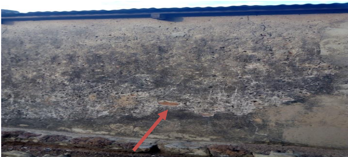
Figure 3h: Plate 8: Exterior cracked teachers bungalow wall at Wa Senior High Teechnical School
