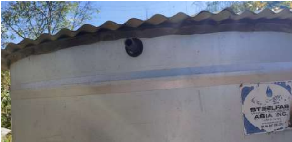
Figure 3. The Water Tank Inlet
