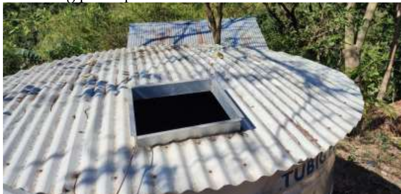
Figure 2. The Water Tank top with Missing Cover (Photo credit to Mr. Kristoffer Paul C. Obispo)
