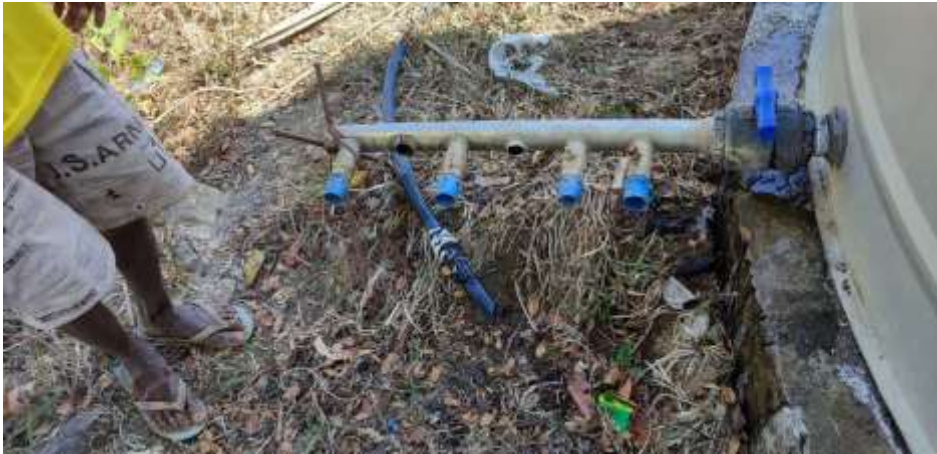
Figure 5. The Water Outlet Distribution Valves (Photo credit to Mr. Kristoffer Paul C. Obispo)
