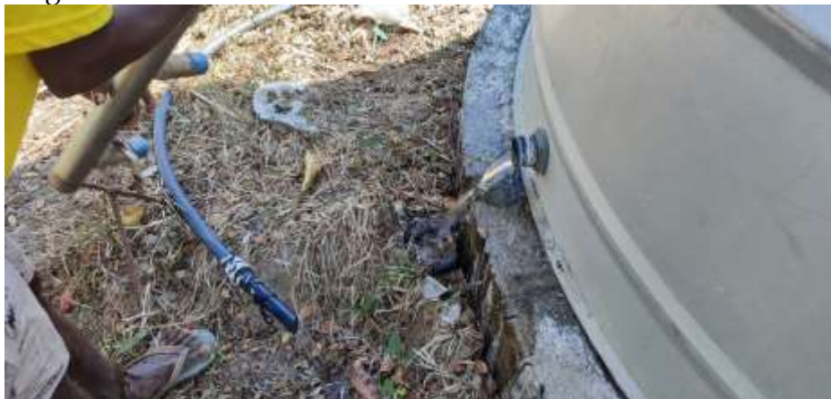
Figure 4. The Water Outlet
