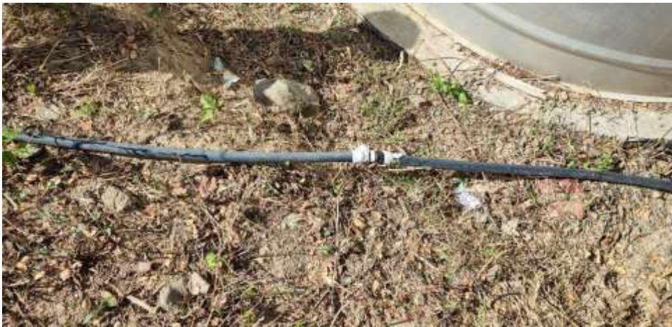
Figure 7. The Water Outlet Alternative Fix (Photo credit to Mr. Kristoffer Paul C. Obispo)
